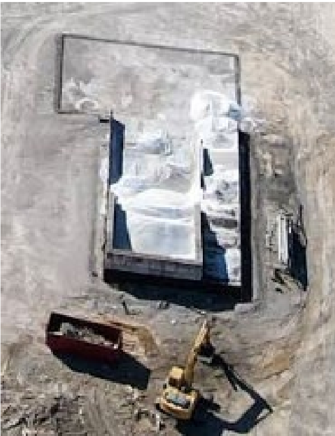
Figure 9. Image from Google Maps of apparent piles of white plastic pellets in open air at the Alpek-Eastman Plant.
