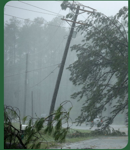
Power lines blown down by Hurricane Florence. Photo by Chip Somodevilla/Getty Images.
