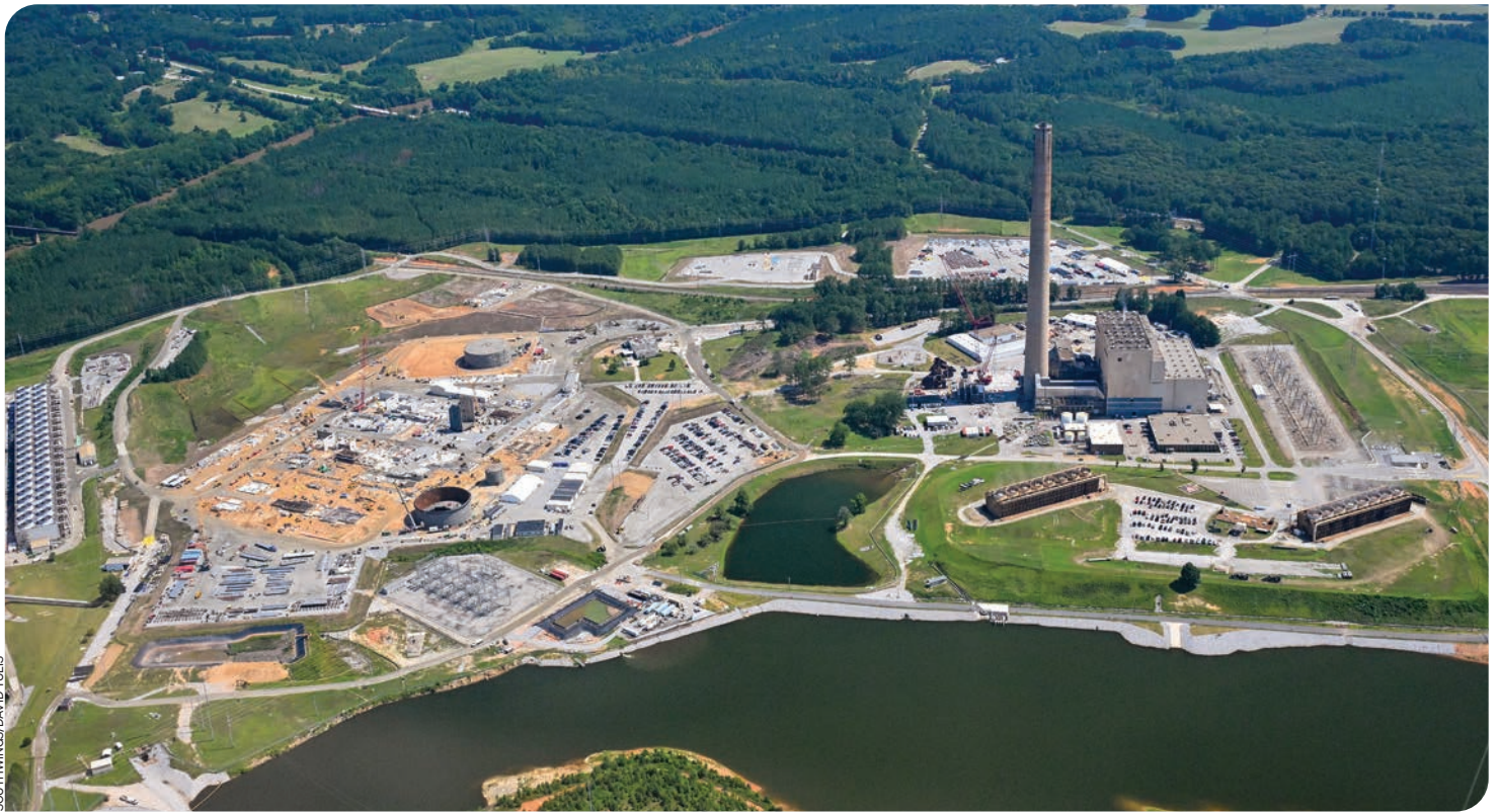
Georgia Power's Plant Yates. An existing 700 MW gas plant is visible on the right; construction of three new combustion turbines is visible on the left.
